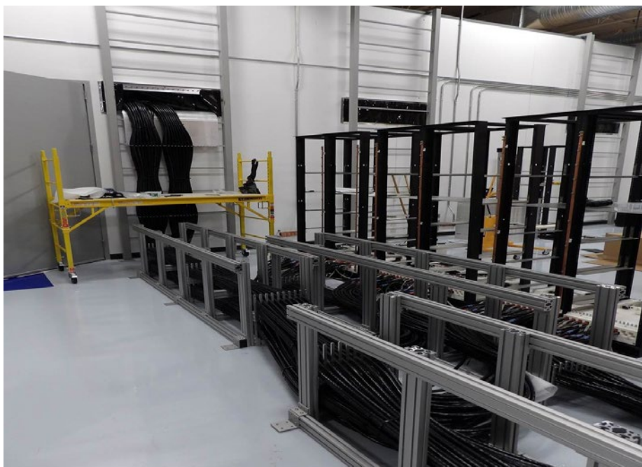
The cabling between capacitors and the flashlamps in the test lab.
